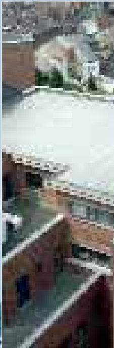
Project: Sint Joseph Hospital (Mons, Belgium, 1992) Product: AlkorPlan® A (Adhered, 3,500 sqm) Old waterproofing: bitumen
